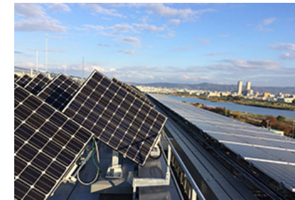
Solar power generation system has panels that move to track the sun's position (at TIC)
